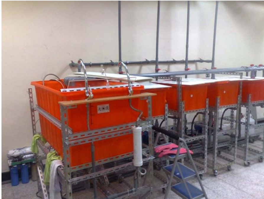
Figure 2. A model plumbing system with goose neck faucets and a Nephros filter
